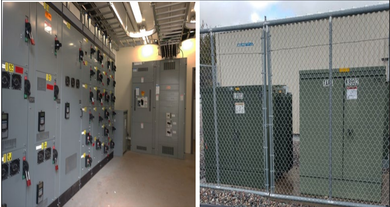
Figure 18-9 Electrical utility plant and transformers
