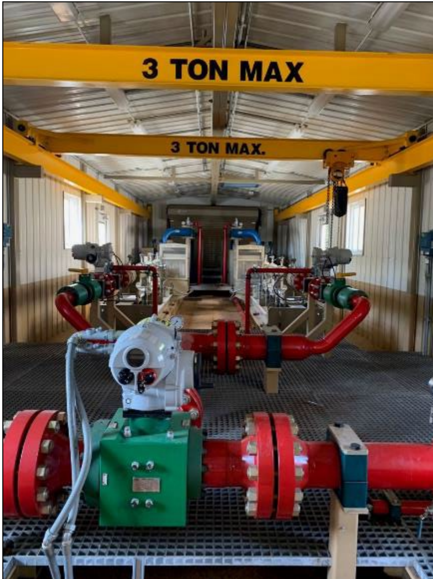
Figure 18-6 Pump building equipment
